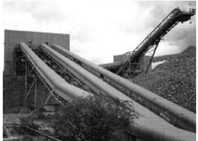
Sprag Clutch holdbacks are often used on inclined conveyor headshaft drives to prevent runback in the event of a power failure.
